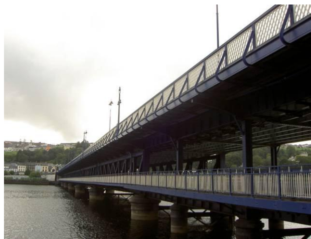
Figure 8. Detail of the "Craigavon Bridge" placed in Londonderry (Northern Ireland) over the river Foyle.
