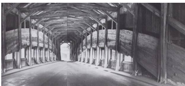
Figure 10. Sight of the wooden bridge constructed in 1839 in Signau (Berne), over the river Emme.
